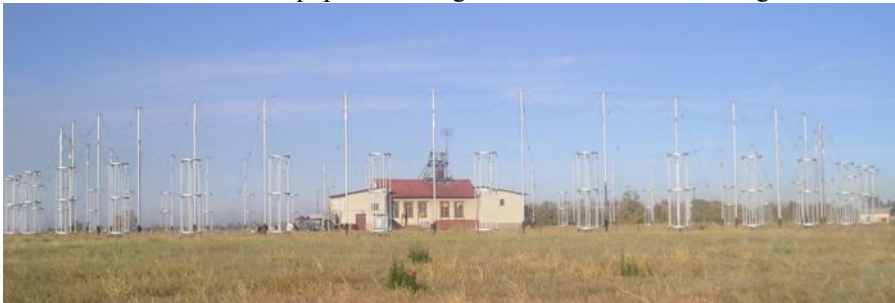
General view of equipment arrangement of RDF station "Krug-M-A"
