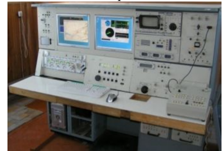
WS of station operator
