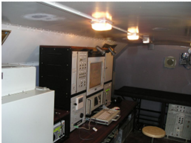
Operators' workplace in the truck mounted container
