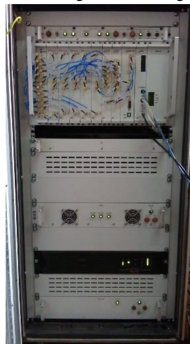
Rack of receiving and measuring device
