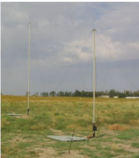
External view of monopoles of DF AFS of “Vostok-RP” station
