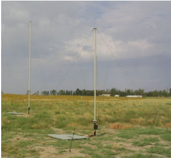
External view of monopole antenna elements of direction finding AFS of "Vostok-RP1" product
