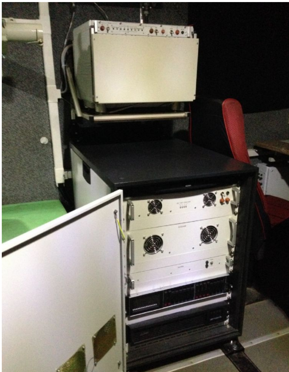
Rack in the composition of the "Barvinok" station
